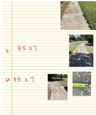
Additional replacement location with larger slab deterioration.
